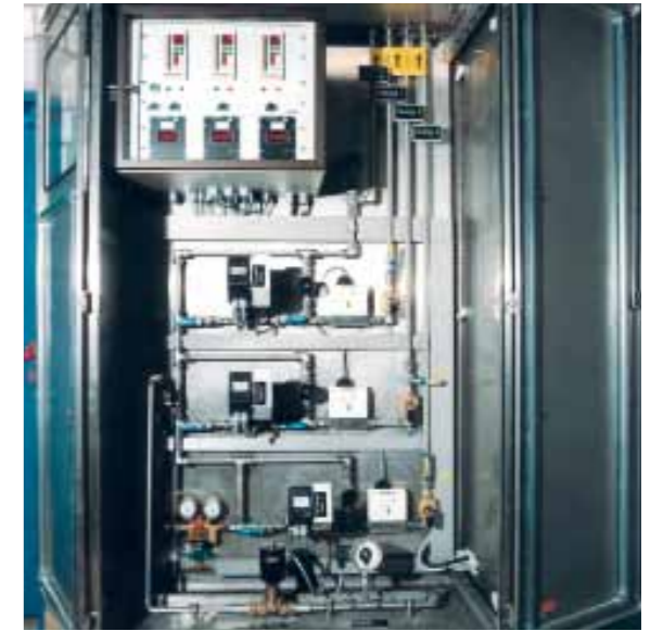
Gas metering unit
