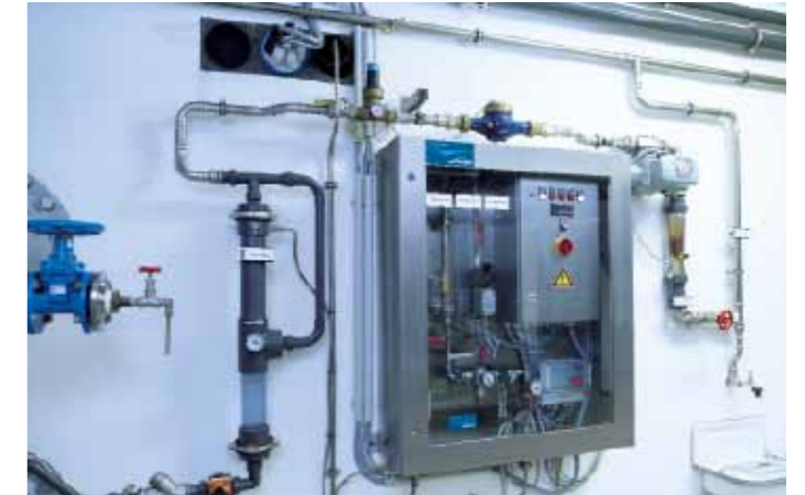
SOLVOCARB®-R reactor with CO 2 metering unit
