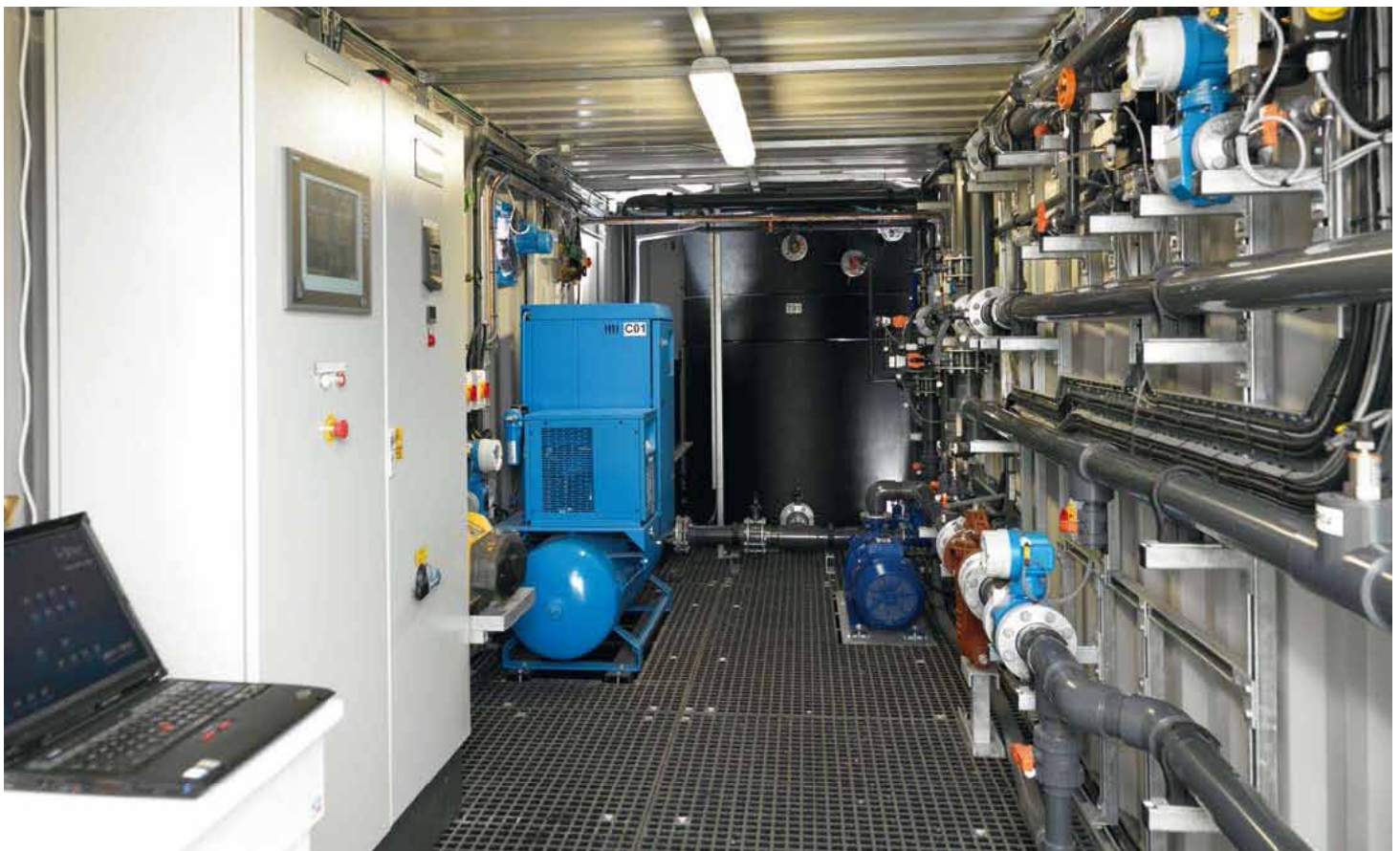
Internal view of the AXENIS™ pilot plant
