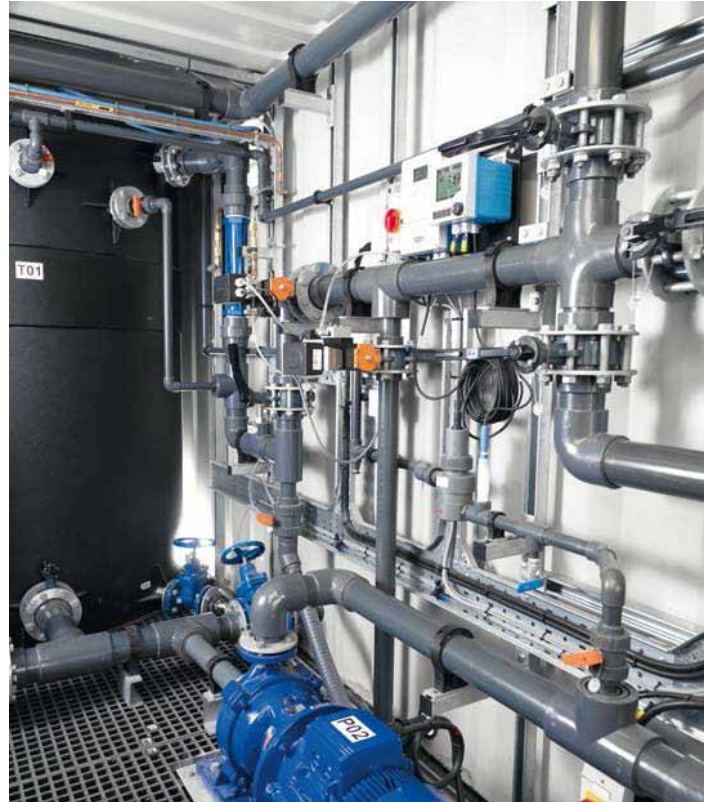
Bioreactor and membrane sidestream pump
